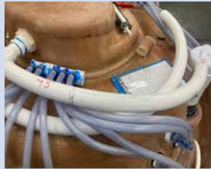
FIGURE E: Right side of spa/step view- Suction and Return lines positioned under Diverter Valve lines for pump hookup/Cardinal pool connection
